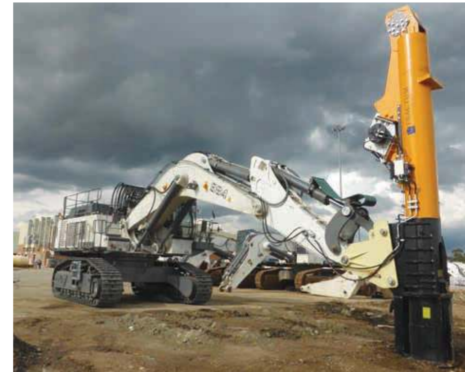
A Fractum 200 fitted to a Liebherr 984 excavator working at an iron ore mine.
